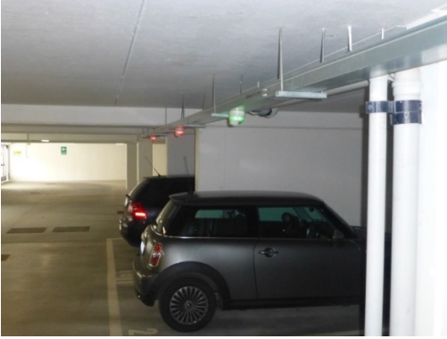
Sensors mounted on the ceiling
