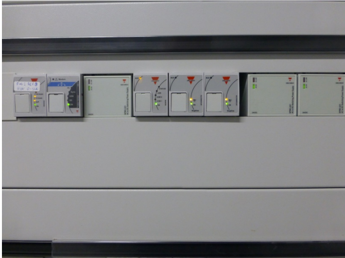
This example shows one SBP2WEB24 and two SBP2MCG324 with two power supplies. To the left we have a display interface module and one SBP2CPY24 that is powered from one power supply
