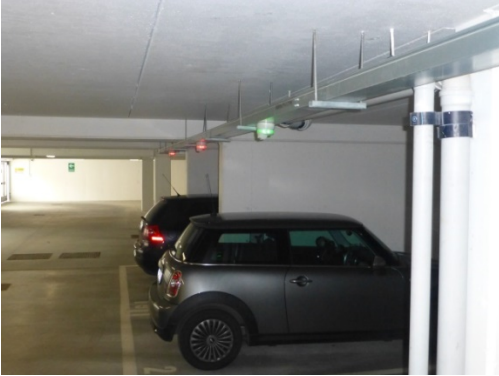
Sensors mounted on the ceiling
