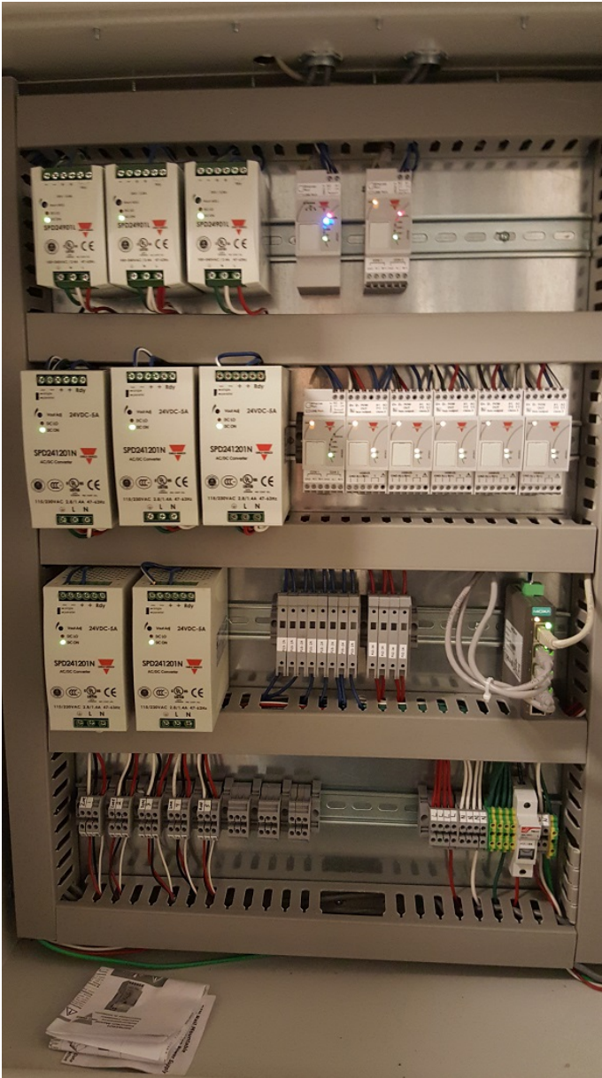
Example of a simple wiring in a cabinet
