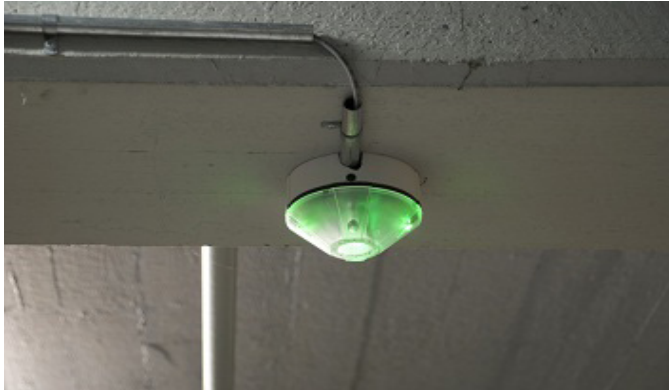
Fig. 35: Sensors mounted on the ceiling
